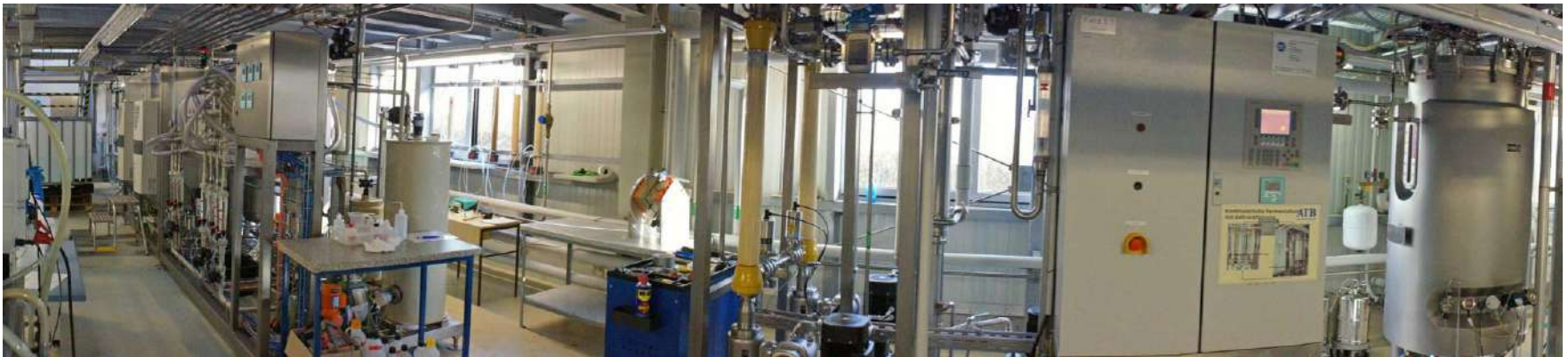
Pilot plant facility for lactic acid fermentation at Leibniz Institute for Agricultural Engineering and Bioeconomy (ATB Potsdam)
